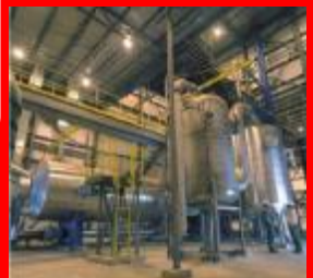
Oil condensing towers
