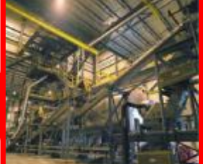
CBpES recovery system
