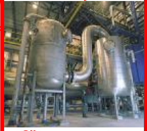
Oil recovery system
